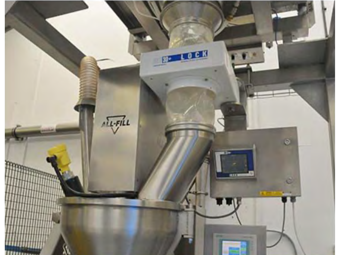
FROM A BIN DISCHARGE TO INTERMEDIARY HOPPER
