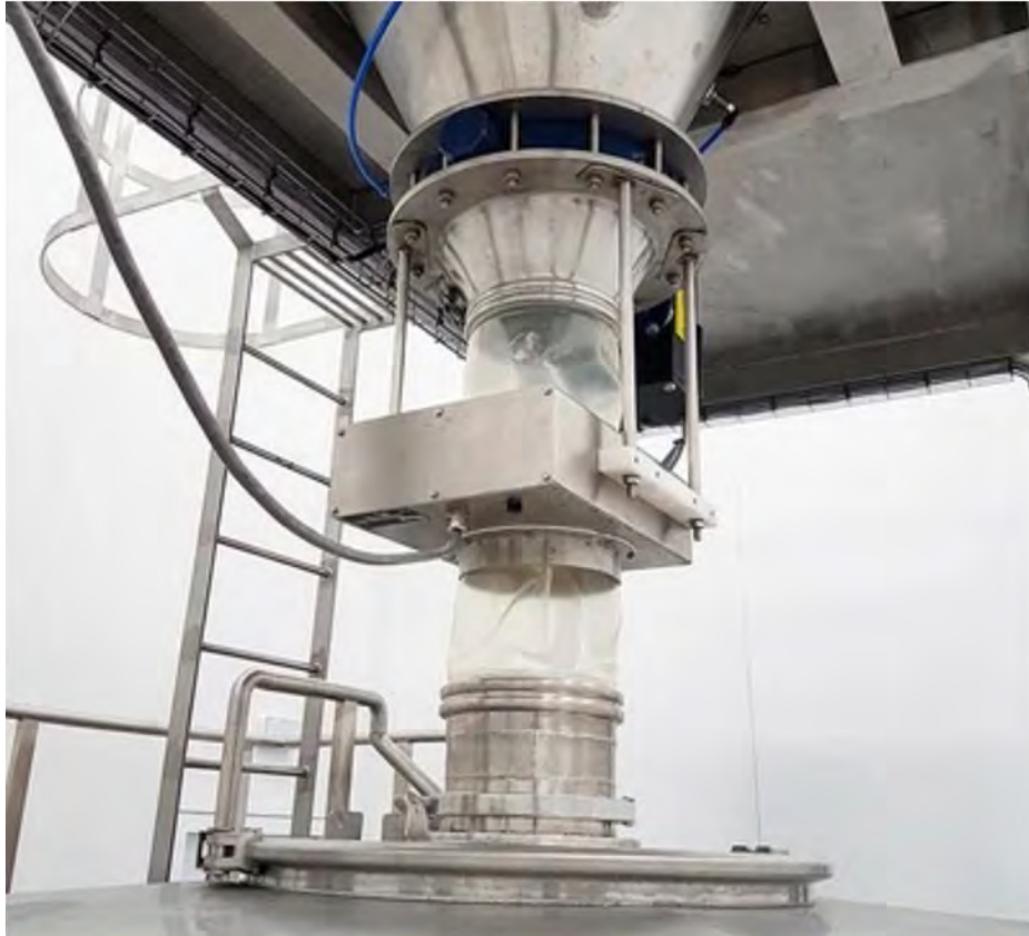
METAL DETECTOR UNDER SILO
