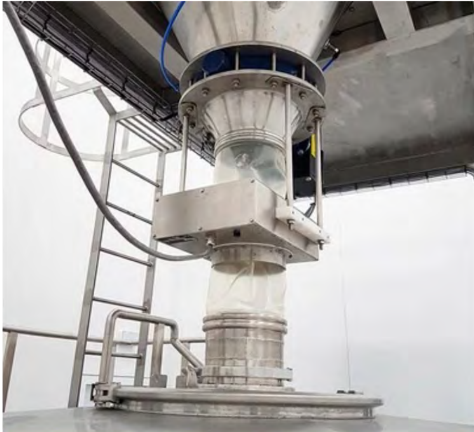
METAL DETECTOR UNDER SILO
